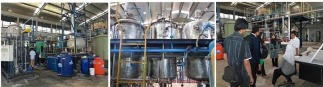
Production of biodiesel at BRDST BPPT Puspitek Serpong with capacity 1 ton BDF per day
